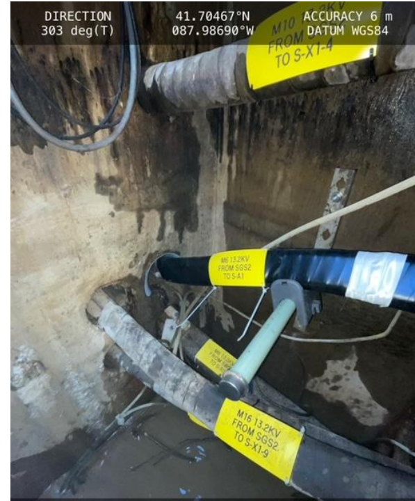
M-6 in MH-3 and cable labeling
