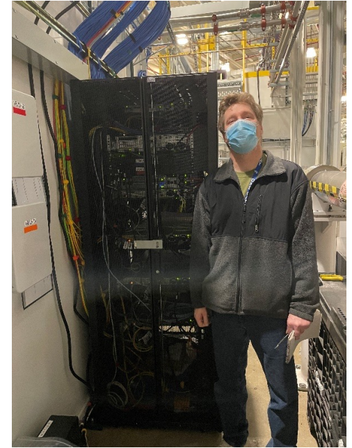
S16 network isolation boxes
