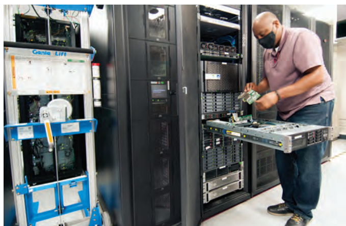
Arista Thurman III, AES Information Technology Group Principal Computer Engineer: “I’m replacing a failed cache module on an SAS disk controller in a DL380 G8 server in the injector control room after component failure resulted in a server being disabled/off-line.”
