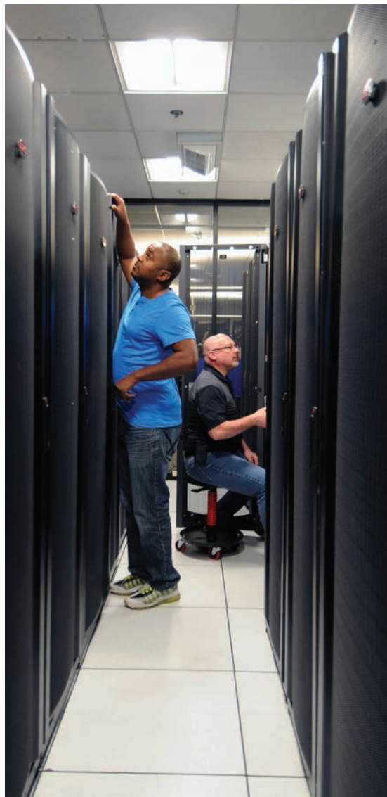
Part of the APS computer room, where servers for the electron storage ring and x-ray beamlines are located.
