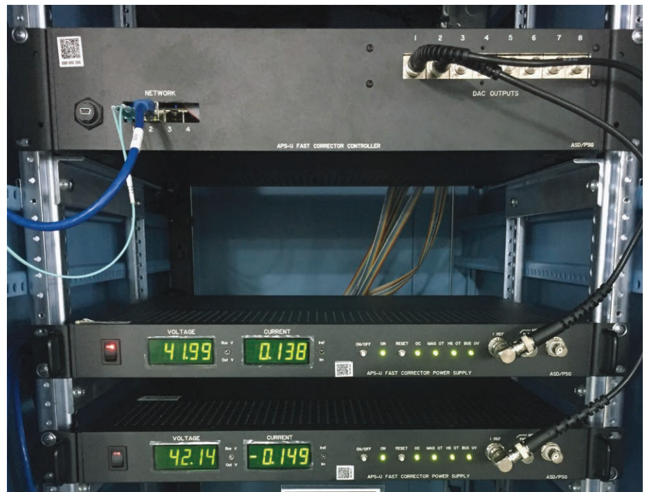
Fig. 2. A bipolar power supply controller and two fast corrector power supplies installed in Sector 27 for APS-U integrated beam stability R&D.
